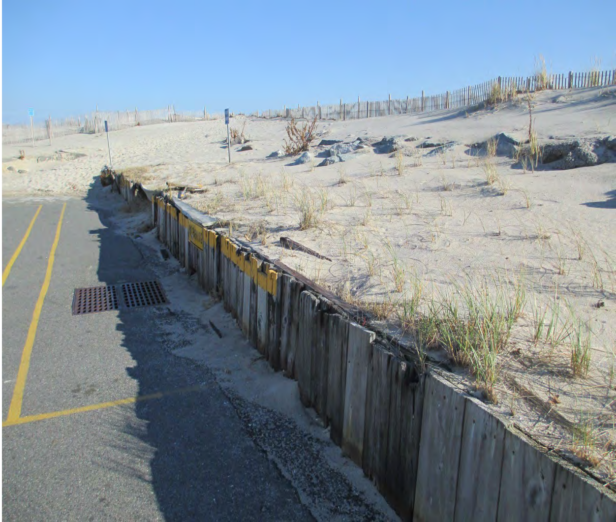
Figure 15: County Bulkhead along Beach Avenue to be Replaced
