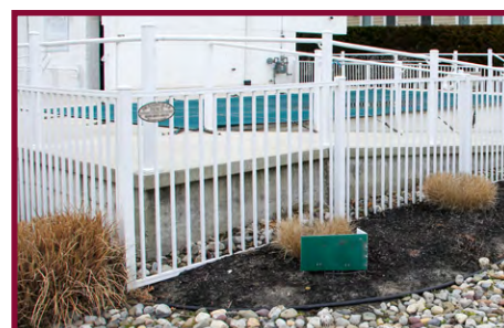
✗ Inappropriate thin aluminum fence and railing
