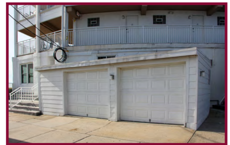
✗ Inappropriate aluminum or vinyl garage doors on a contributing building
