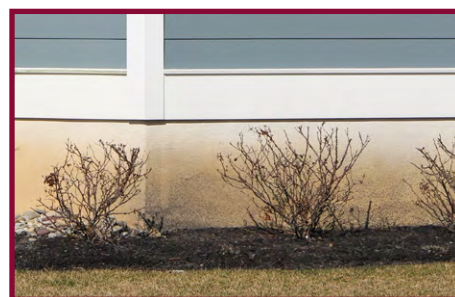
✗ Inappropriate exposed concrete foundation
