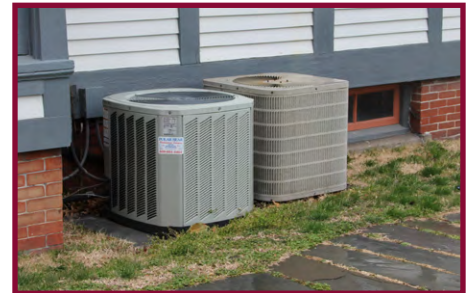
✗ Inappropriate visible mechanical equipment without screening
