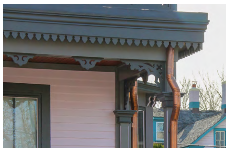
Copper gutter leaders
