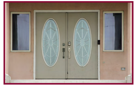
✗ Inappropriate front door
