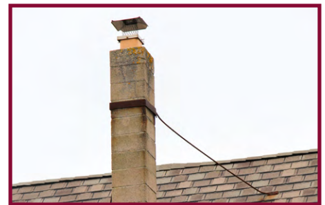
✗ Inappropriate exposed cement finish chimney
