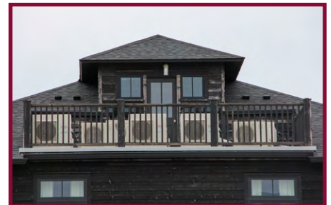
✗ Inappropriate visible mechanical equipment partially screened
