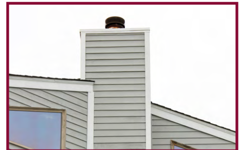
✗ Inappropriate chimney clad with siding
